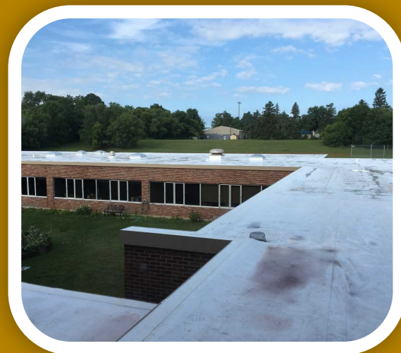
The new roof of the academy, keeping the rain from leaking through the ceiling into the classrooms
