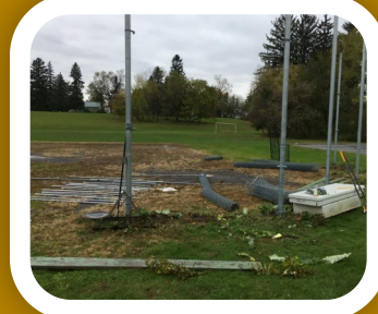
The baseball backstop coming down to make room for the new parking lot
